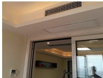
Central air conditioning
